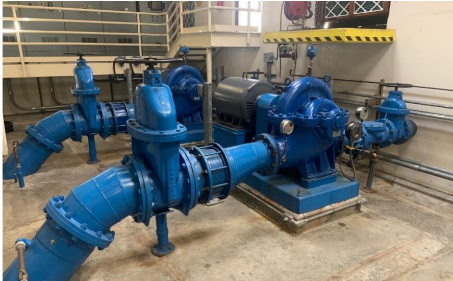
Figure 1: Whisman Pump Station – Pumps 1 and 2
