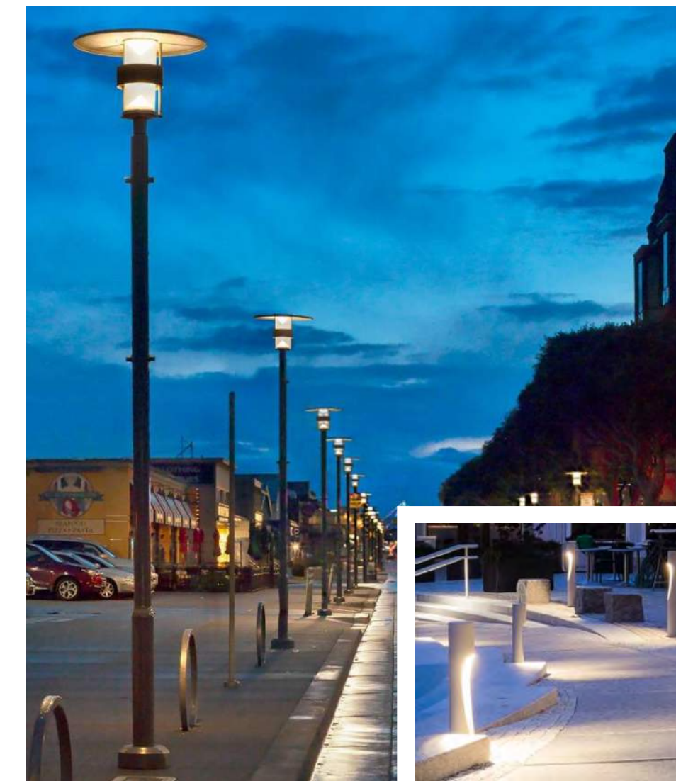
Pedestrian Pole Lights and Bollard Lights
