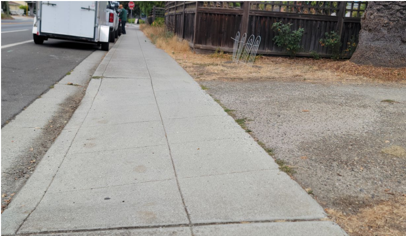
Figure 9 Example of a Non-Compliant Sidewalk
