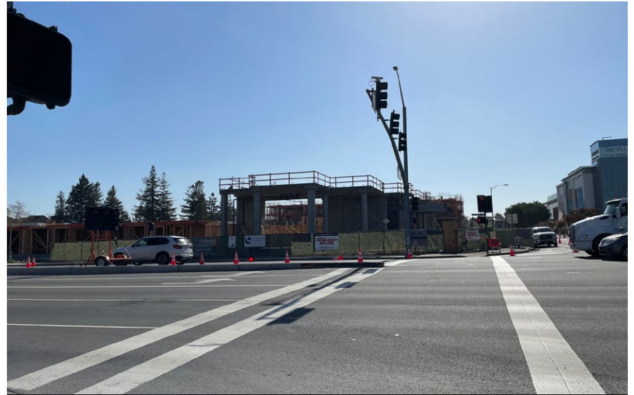
b. View of construction site facing east immediately north of the Project site across California Street.
