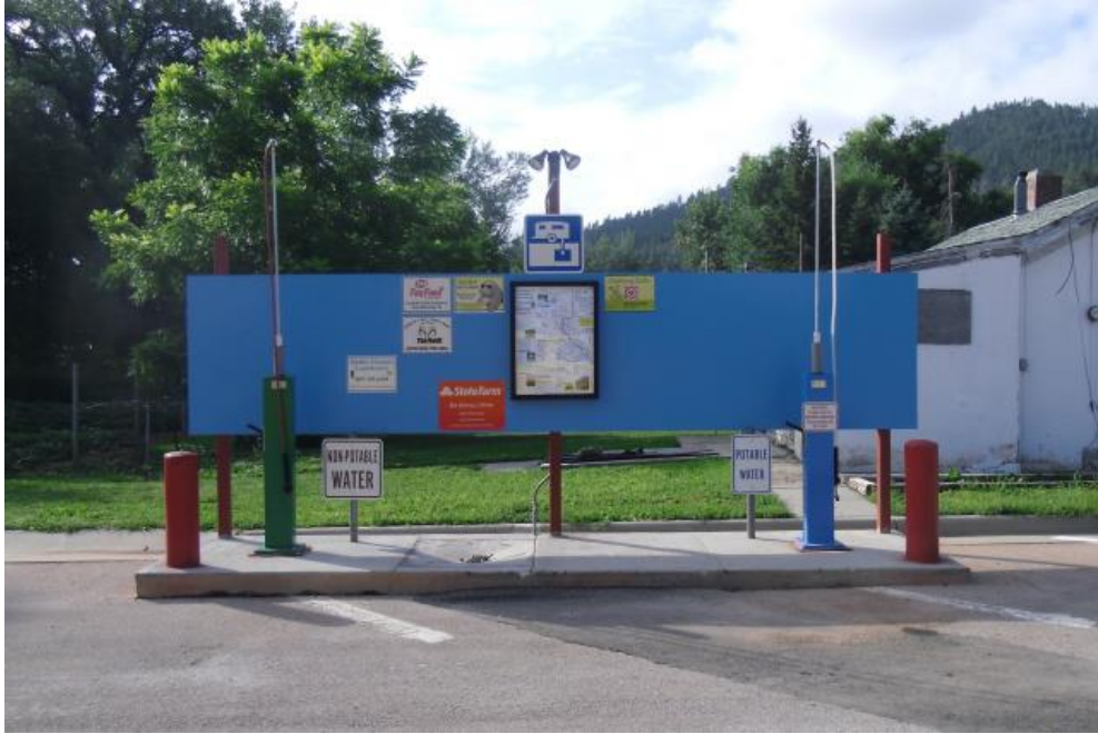
Figure 1 – Dump Station with Waste Disposal and Water Towers in Raised Concrete Pad
