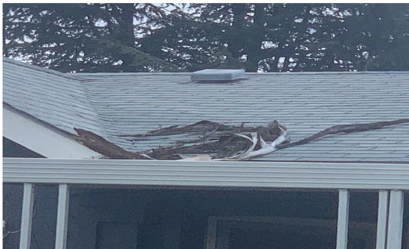
Figure 3 (Debris on roof)
