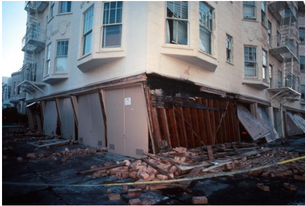
1A. Near-collapse, San Francisco, Loma Prieta earthquake
