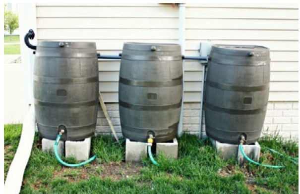
Rain barrels facilitate stormwater management
