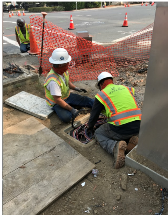
Figure 7: Signal Infrastructure Upgrades Being Completed as Part of a Development Project
