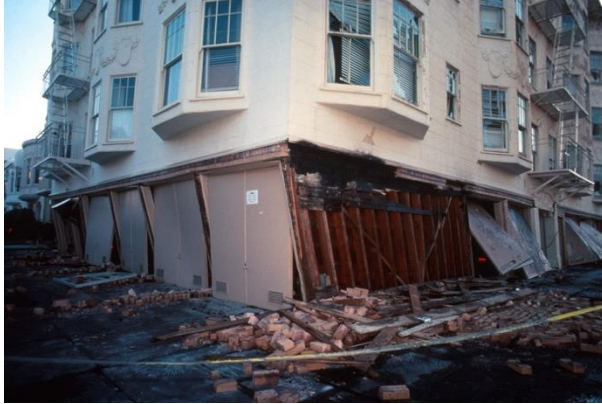
Near-collapse, San Francisco, Loma Prieta earthquake
