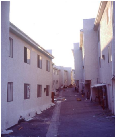
Left: Collapse. Right: Sidesway damage, Los Angeles, Northridge earthquake (Credit: Gary D. Avey)
