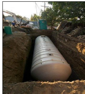
Figure 2-9: Cistern at private residence in Mountain View. (Source: Vox Design Group)
