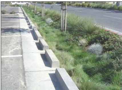
Figure 2-1: Bioretention area capturing parking lot runoff, San Jose (Source: City of San Jose)
