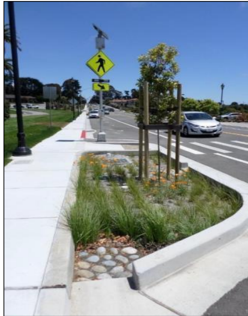
Figure 2-10: Bioretention incorporated into bulb-out designed to improve pedestrian safety. (Source: EOA, Inc.)
