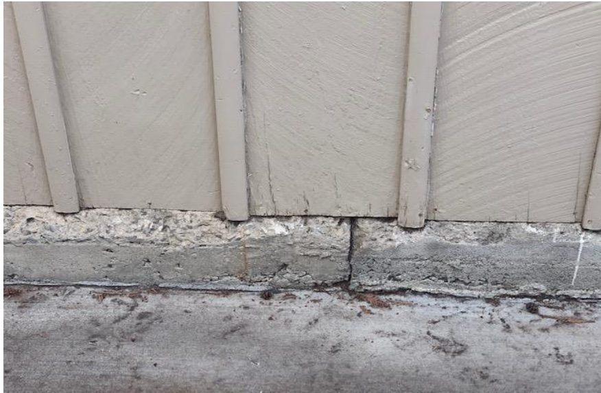
Figure 5: Compromised Section Concrete Slab
