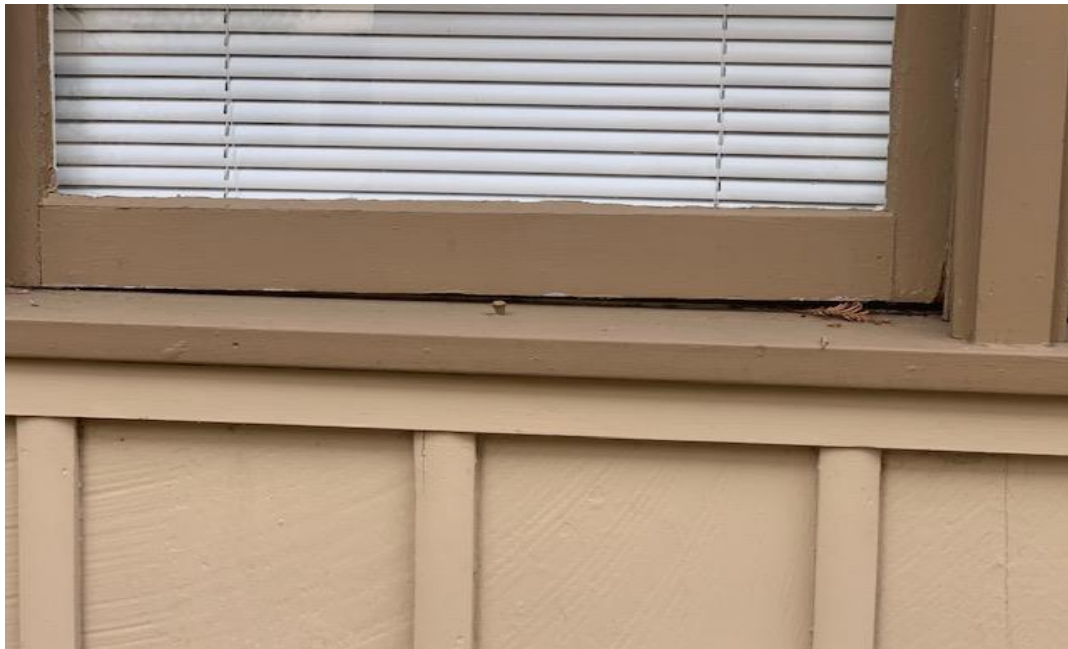
Figure 4: Gap in Window Closing
