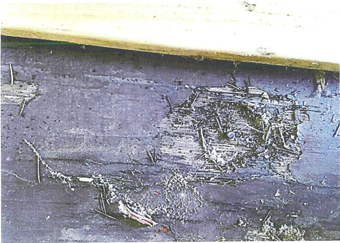
Repair damage to plywood surface at second floor walkway.
