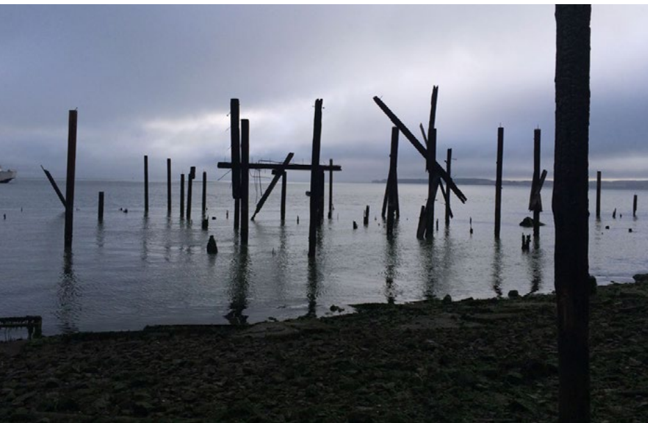
Creosote-treated pilings at the Red Rocks warehouse site in Richmond. Photo by Marilyn Latta, State Coastal Conservancy.
