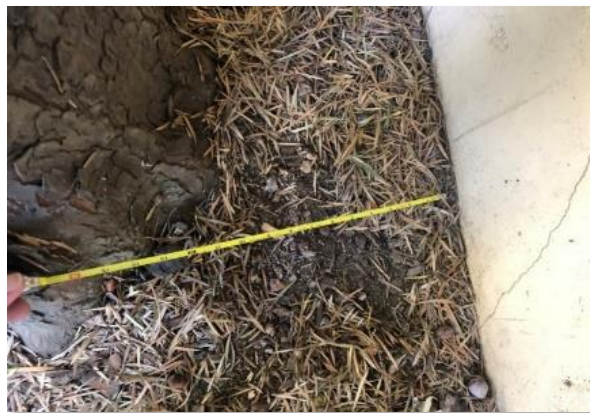
Figure 3: Tree No. 1 Proximity to Wall
