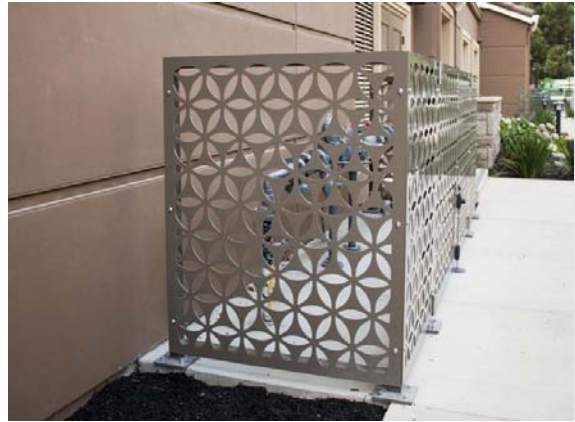
Decorative screening to minimize the appearance of utilities
