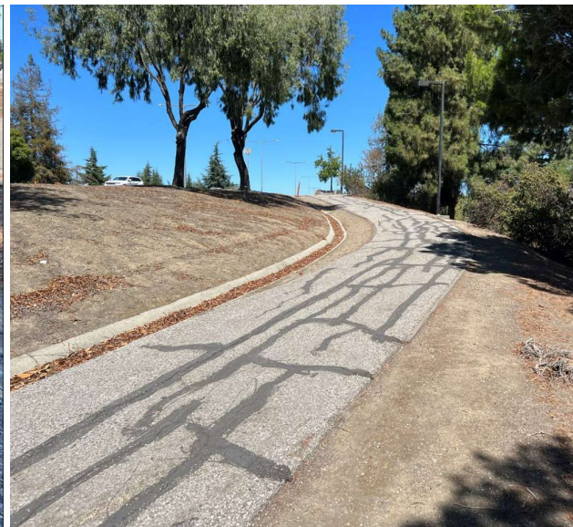
Figure 2: Existing Steep Slope Condition
