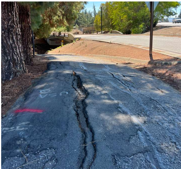
Figure 1: Existing Poor Asphalt
