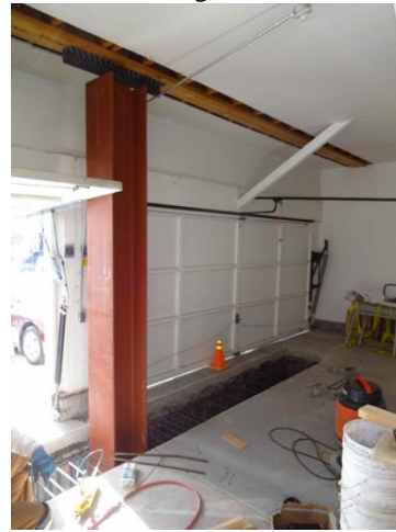
Cantilever column installed with new concrete footing (awaiting concrete) (Credit: Thor Matteson)
