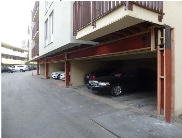
Three-bay steel moment frame installed around garage door openings, with new concrete footing (Credit: Degenkolb Engineers)
