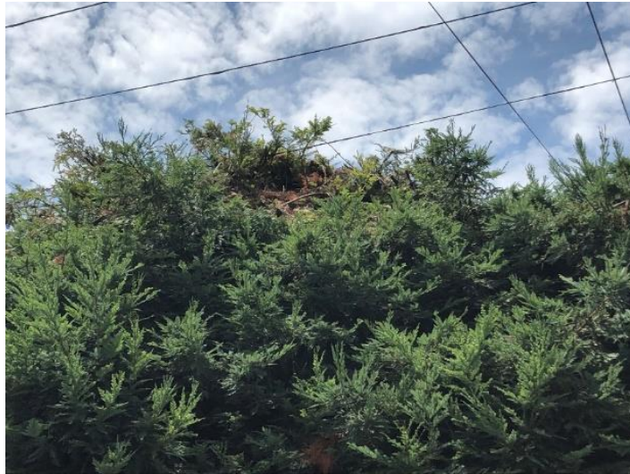
Figure 3: Tree Proximity to Secondary Lines
