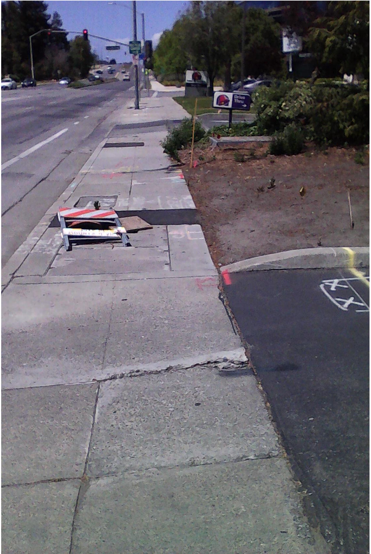
Datavisor to Taco Bell. Tilted sidewalk, plywood and flopped-over warning sign covering open excavation.
