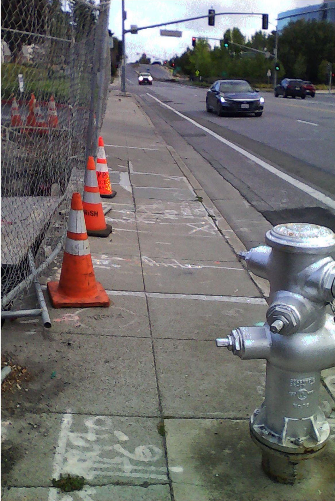
Approaching 1215 Terra Bella. 6' sidewalk, no setback. Hydrant, cones and fencing around open excavation obstruct pedestrians. Views from driveway also bad,
