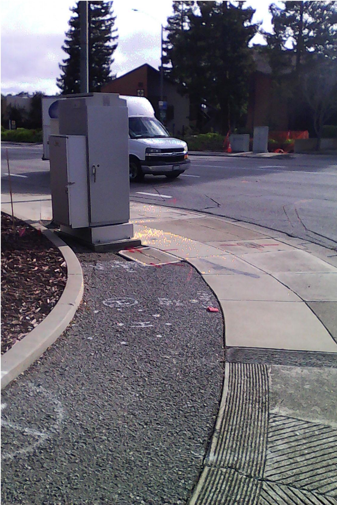
NW corner Shoreline @ Middlefield outside Chevron station. Utility box obstructs pedestrians' and drivers' views
