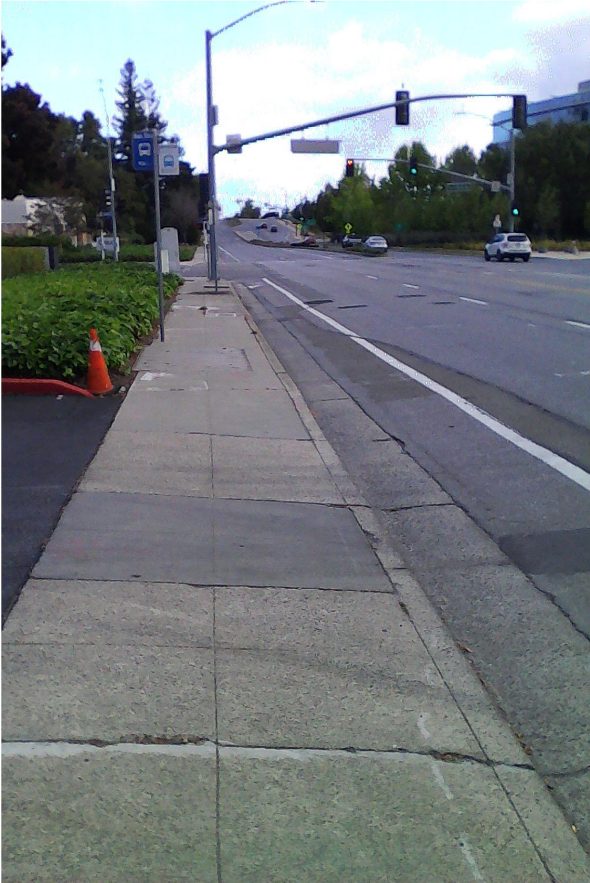
1215 Terra Bella driveway -- 6' sidewalk, no setback. Good place to get run over.
