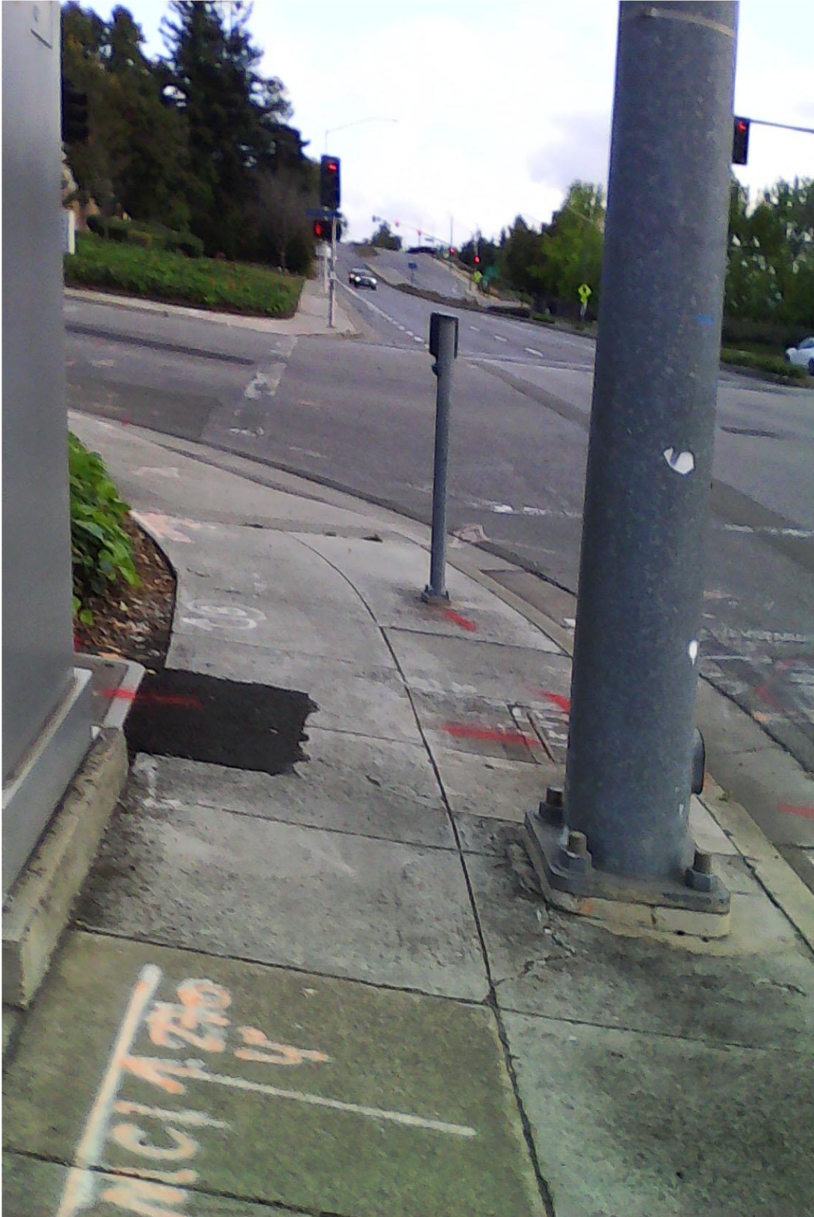
SW corner of Shoreline at Terra Bella 6' sidewalks, no setbacks. Excavation. Pedestrians squeezed by poles & utility box.
