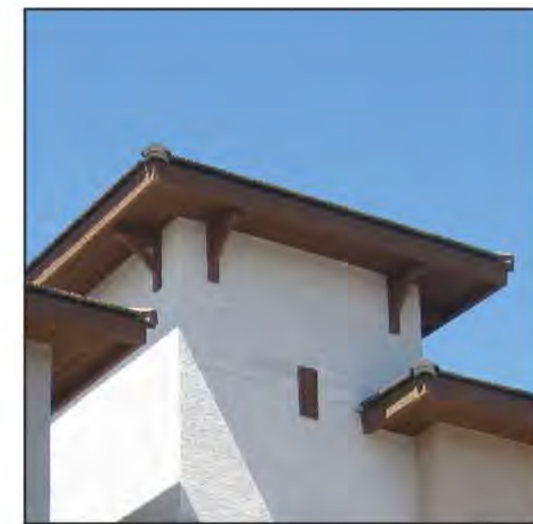
8 ENHANCED ROOF CAP AT EAVE PLASTER OVER WOOD FRAMING PLASTER OVER FOAM BRACKETS
