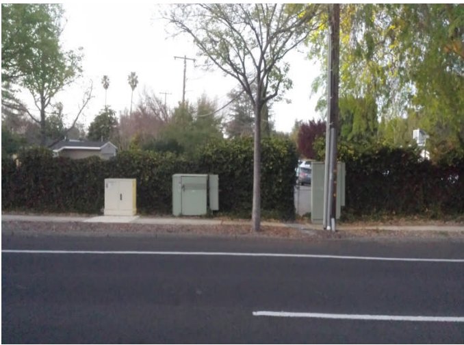
Figure 2-4: Central Expressway East Side, Existing AT&T Utility Cabinets
