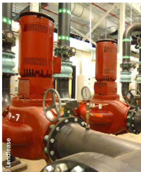
Figure 9.3.1 Interior view of the East Carolina University Central Utility Plant
