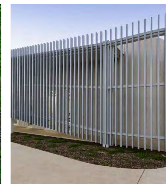
(MF) ALUMINUM METAL FINES @ PARKING GARAGE
