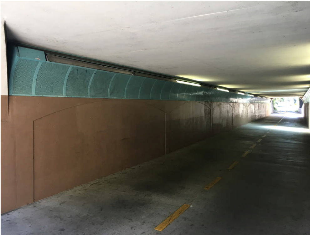
Figure 3-3: Lighting and wall and ceiling colors, Stevens Creek Trail tunnel under El Camino Real, Mountain View
