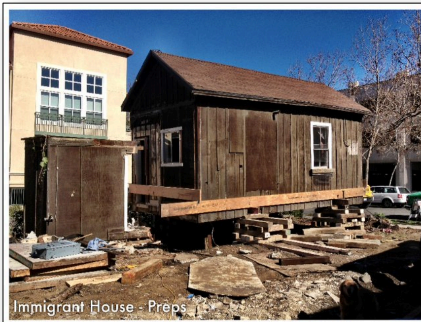
Figure 4 – Immigrant House being prepped for relocation to its temporary location at 231 North Whisman Road. Looking north at the side of the building.
