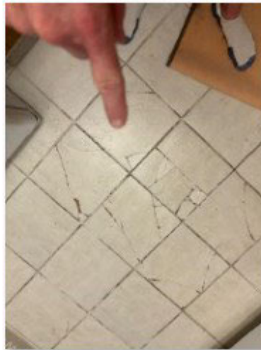
Floor damage, kitchen - Jun 2025 (4)
