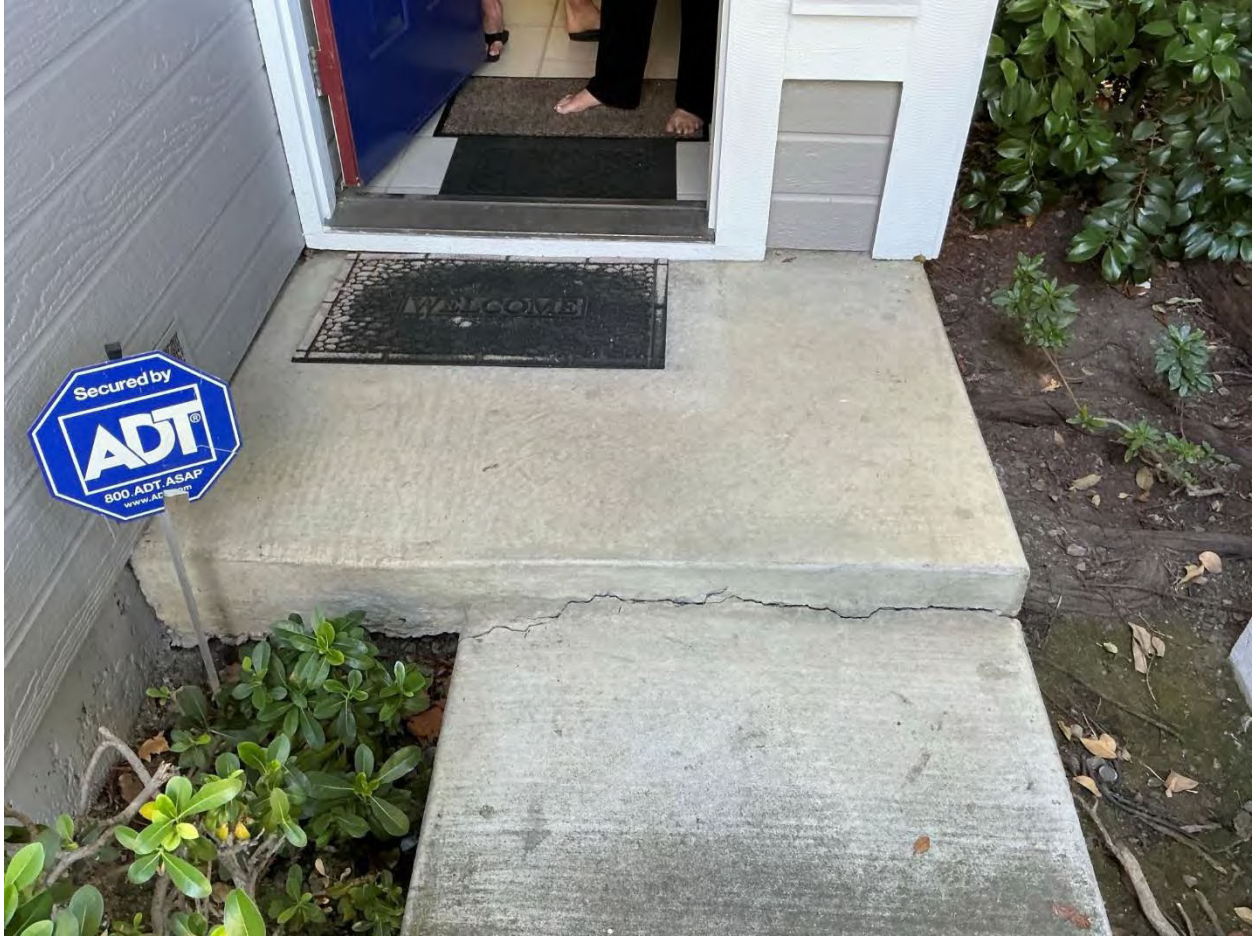
Lifting damage from roots
