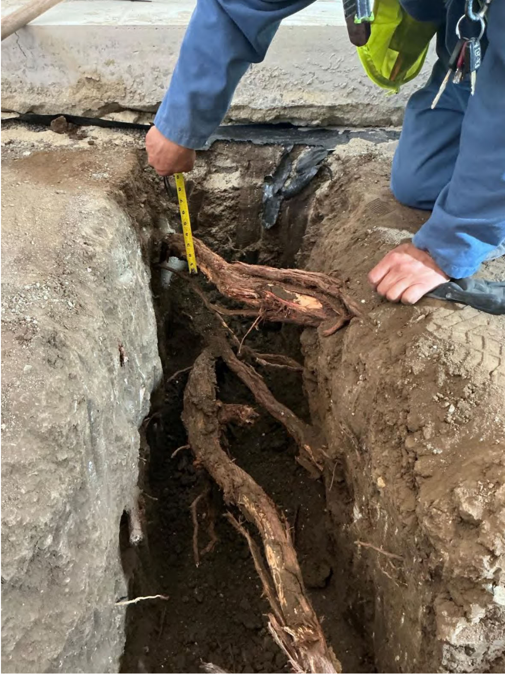
Roots from South Side
