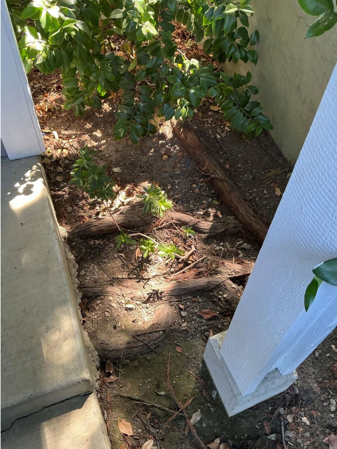
Large Surface rooting at entrance
