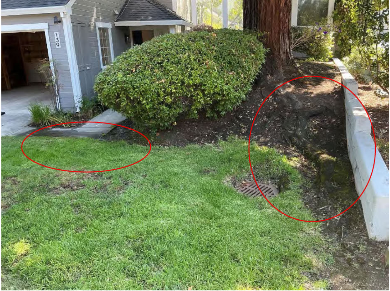
Large Surface rooting, saturated lawn, puddles on walkway
