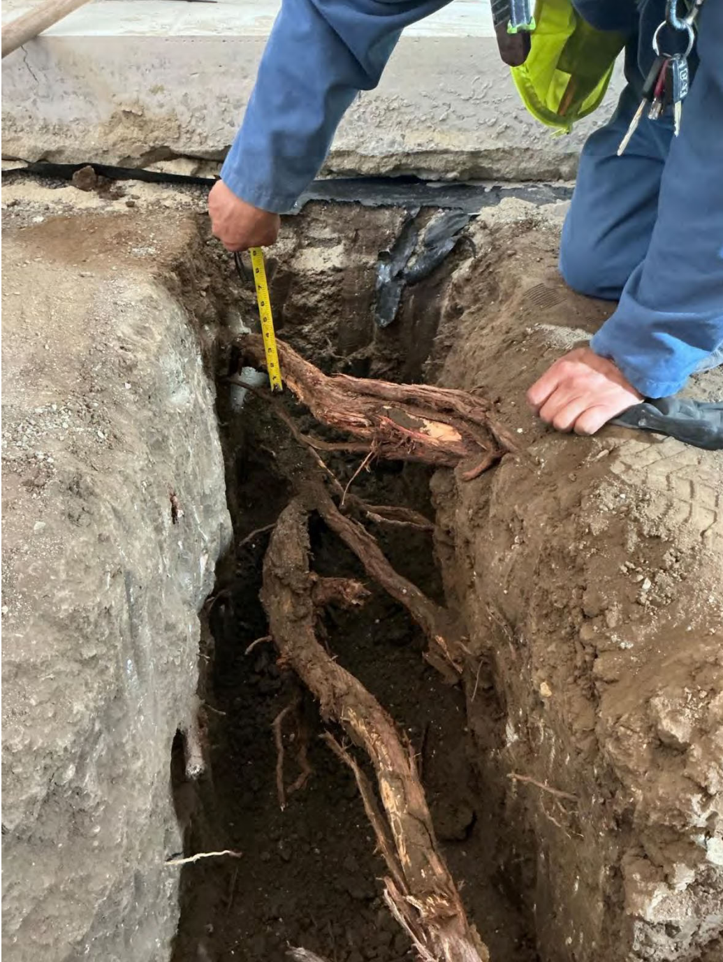
Roots from South Side
