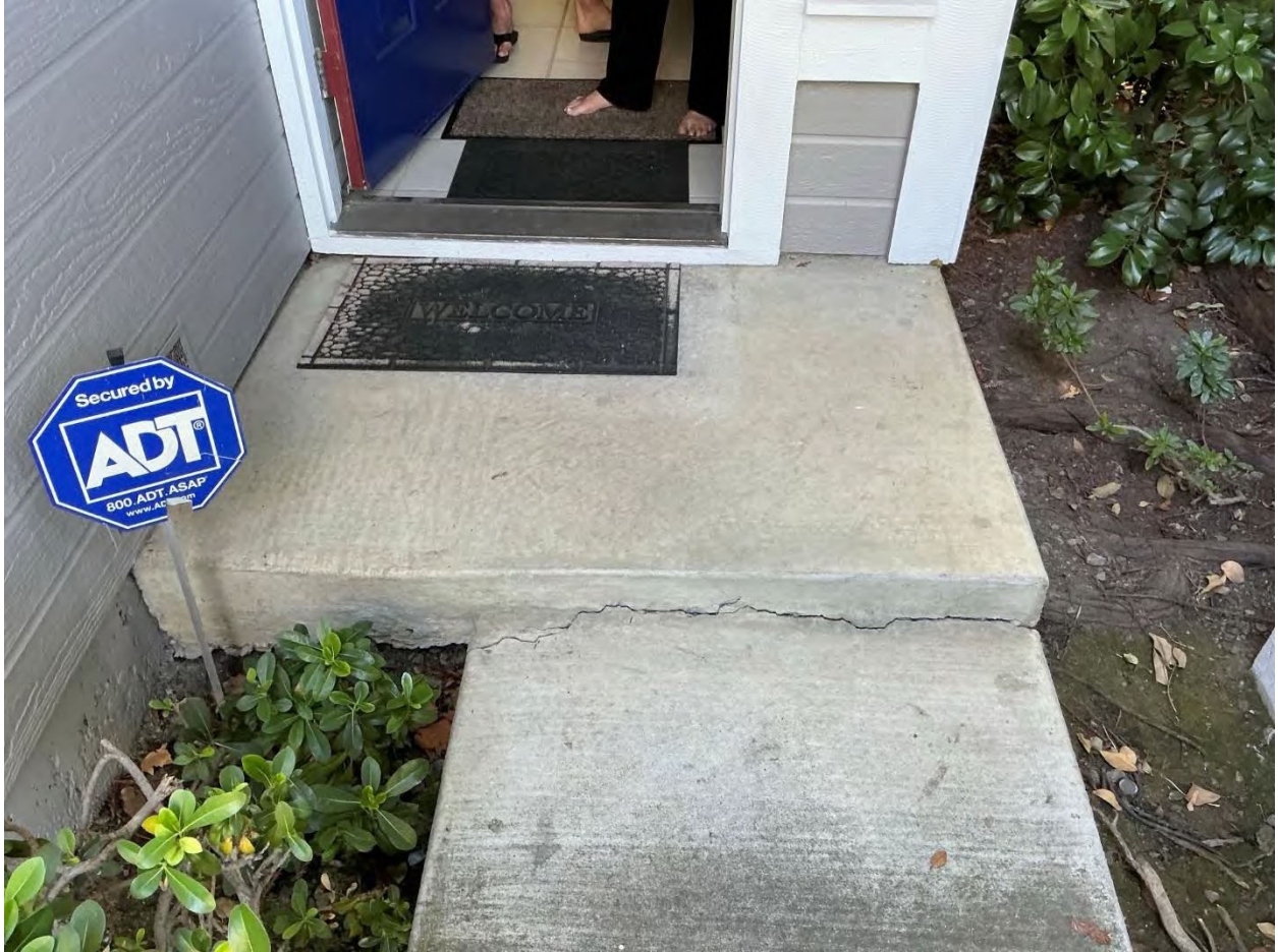
Lifting damage from roots
