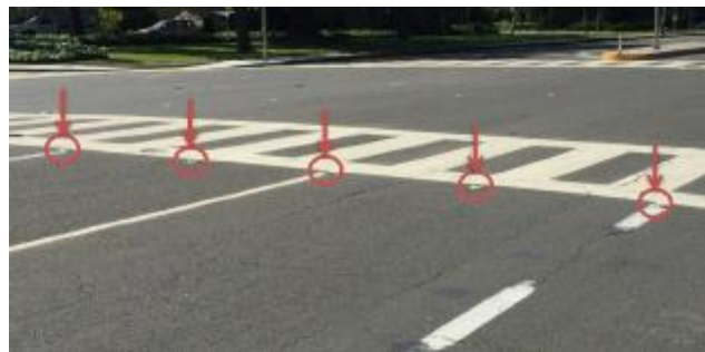
Figure 2 – Example of In-Roadway Warning Lights (IRWLs)
