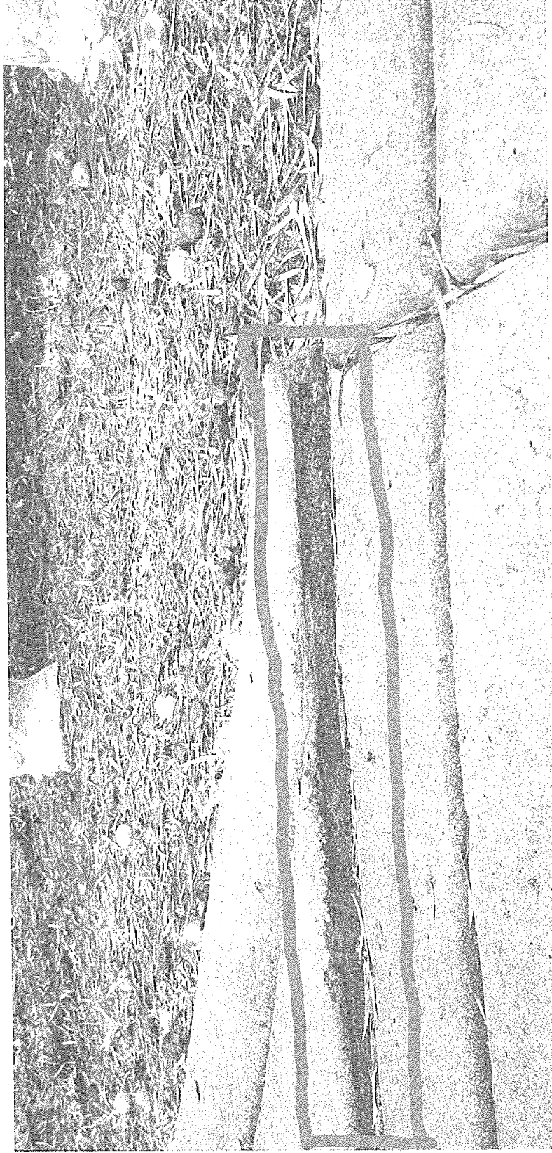
ELMAR GLIBICKY 1100 CARLOS PRIVADA CONCRETE WALKWAY OF PATTO - LIFTED BY ROOTS
