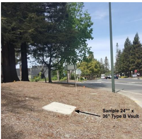
Figure 2: Example of Underground Vault (left) and Above Ground Cabinet (right)
