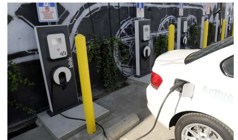
EV charging stations within all parking structures.
