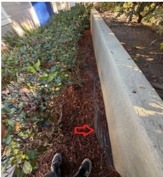
Photo #7 Photo of approximate 4-inch surface root near retaining wall.
