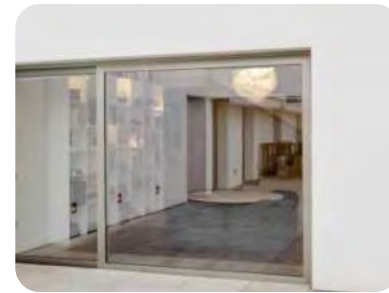
EXISTING SLIDER WINDOWS
