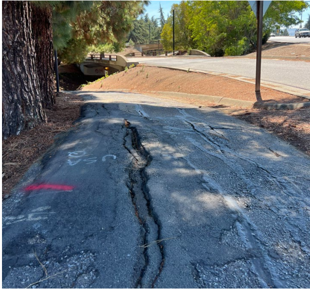
Figure 2: Existing Poor Asphalt
