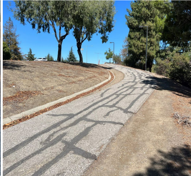
Figure 3: Existing Steep Slope Condition
