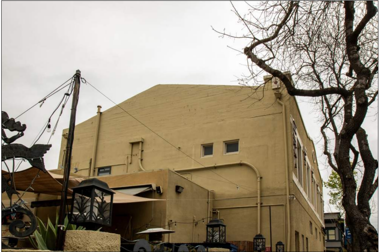
Rear facade showing pointed parapet and board form at top and addition on first floor. The original windows are gone.
