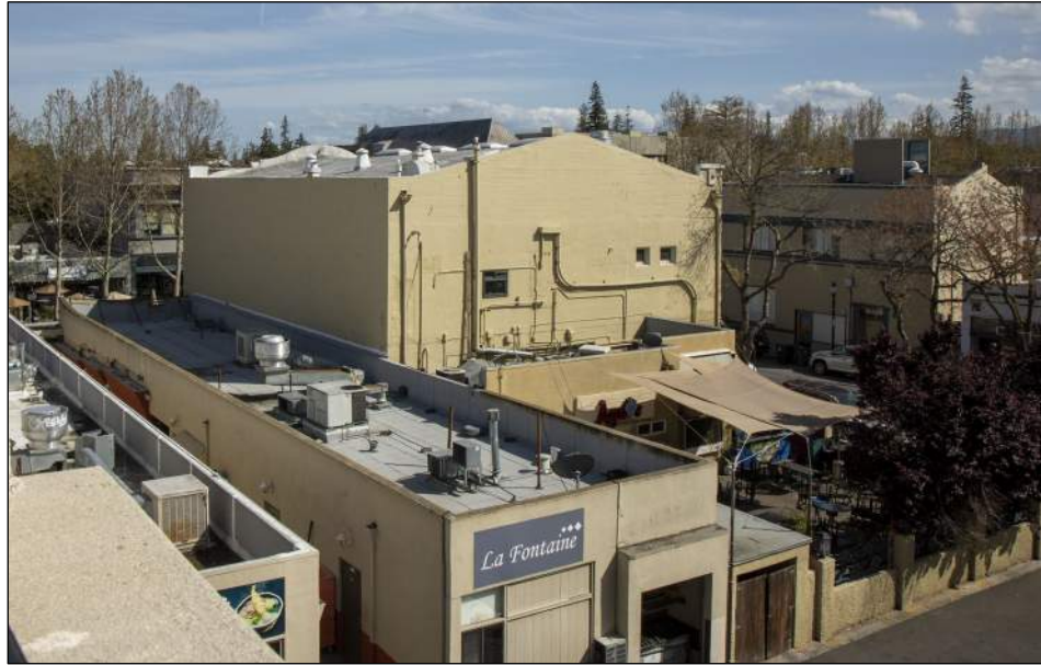
Rear facade viewed with camera facing southeast. The roof of the L-shaped addition is visible as are the modified rear windows.
