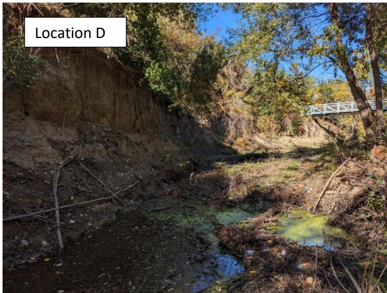
Figure 5 – West bank erosion adjacent to Whisman Park
