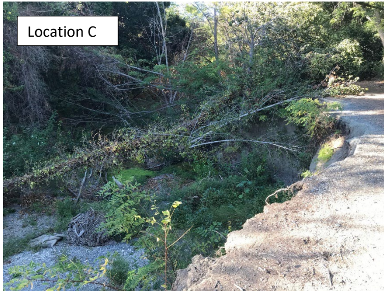
Figure 4 – East bank erosion adjacent to the German International School of Silicon Valley
