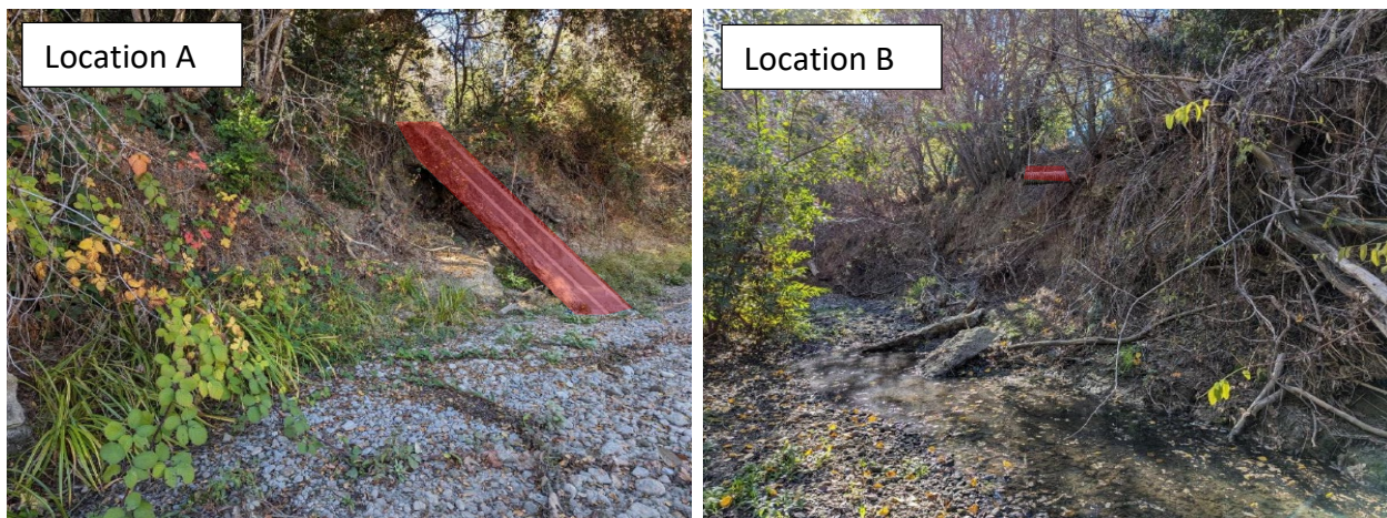
Figure 3 – Erosion around storm drain outlets (red highlight)
