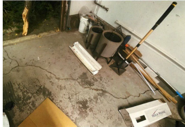
Figure 4: Photo of concrete damage within garage
