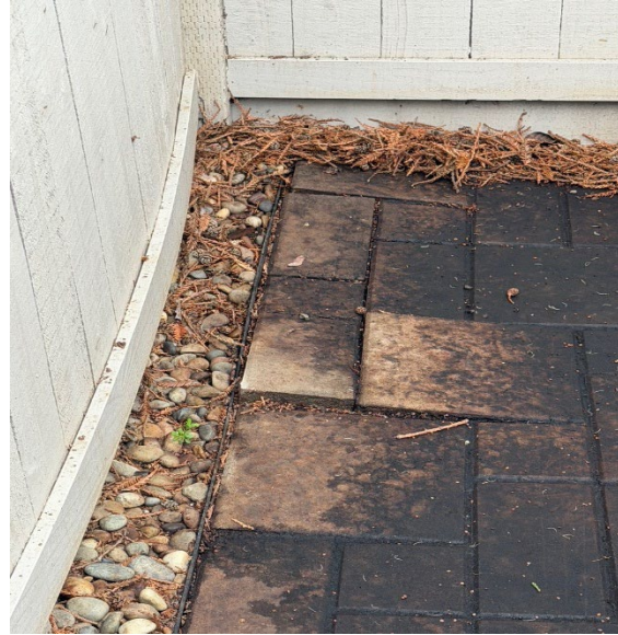
Photo #6 Photo of uplifted of pavers (approx. 1 inch.)
