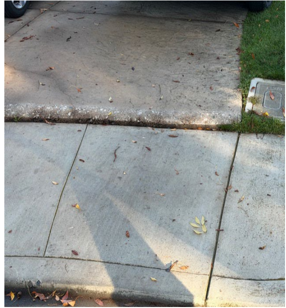
Photo #6 Photo of 3" uplift driveway
