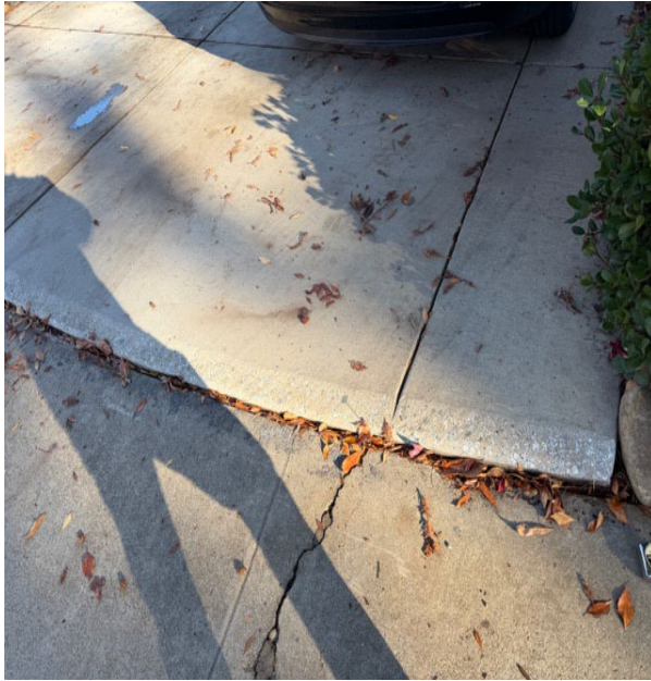
Photo #5 Photo of 2" uplift driveway damage
