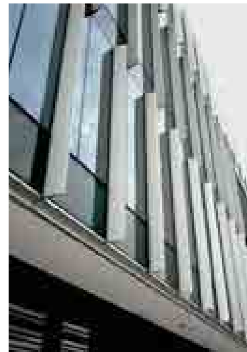
(MF) ALUMINUM METAL FINES @ PROPOSED OFFICE BUILDING
