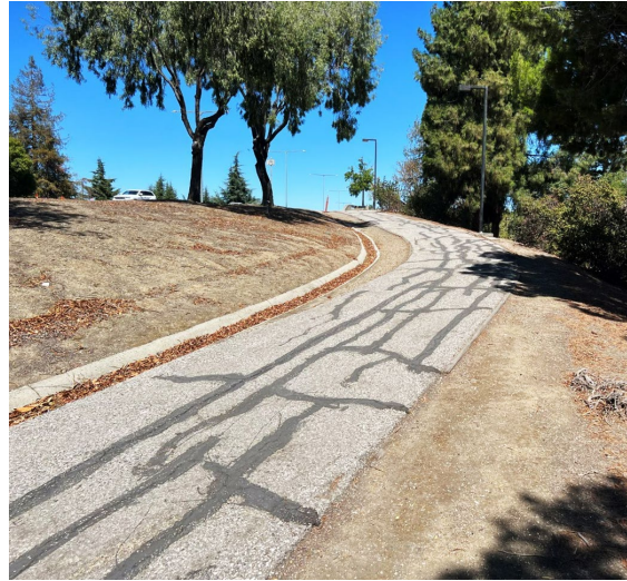
Figure 3: Existing Steep Slope Condition
