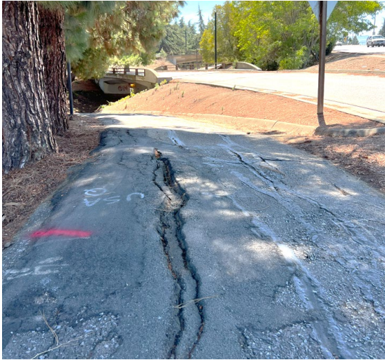
Figure 2: Existing Poor Asphalt
