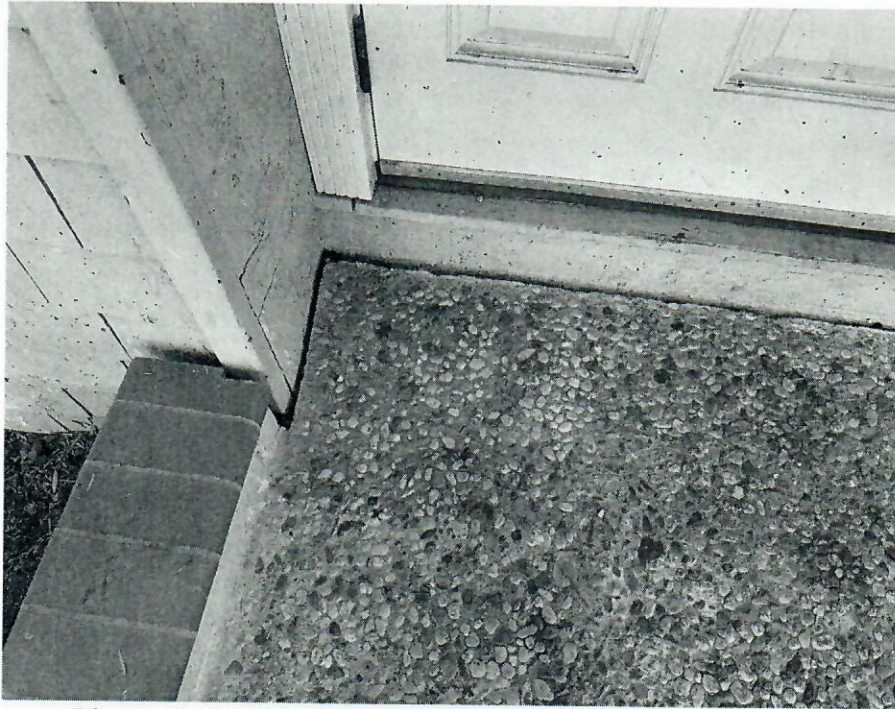
Picture 9: Location of approximately 1" plus gap at landing
