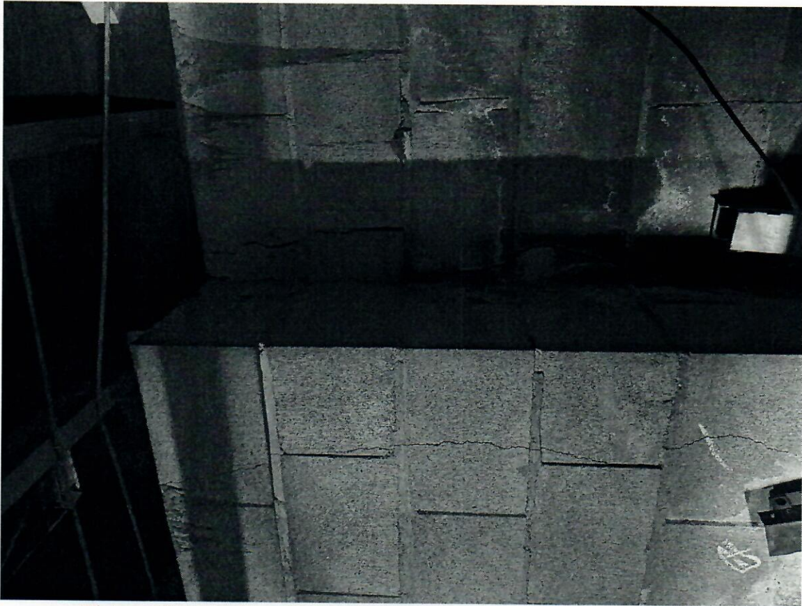
Picture 17: Location of vertical crack at inner face of existing block retaining wall foundation
